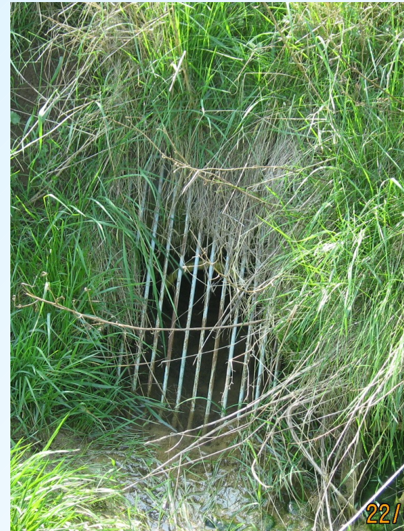
Exit of a drainage collector
