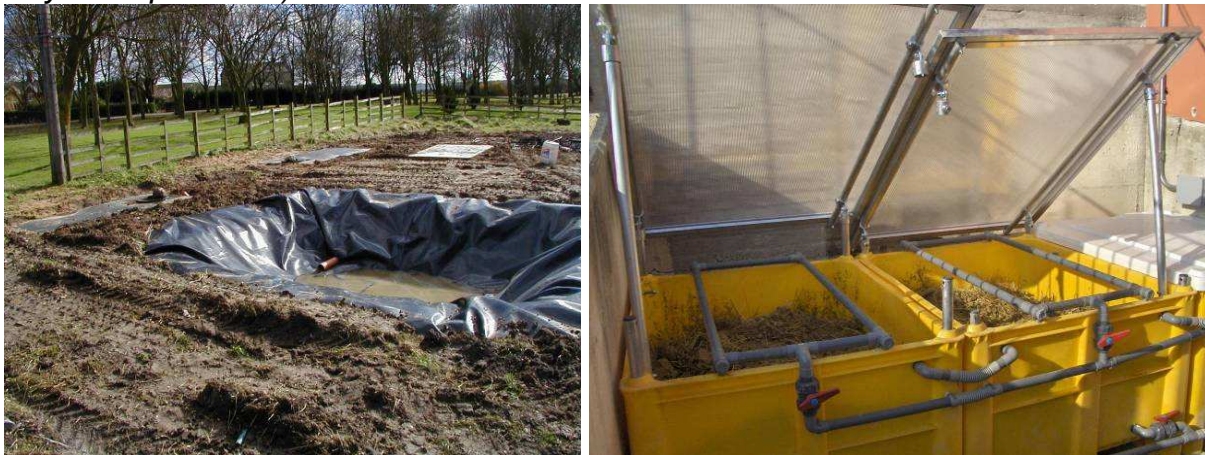
Fig. 25 & 26: As an alternative for concrete, biobed can also be lined with plastics such as EPDM (left, source ADAS) and PE containers (right, source Mybatec).
