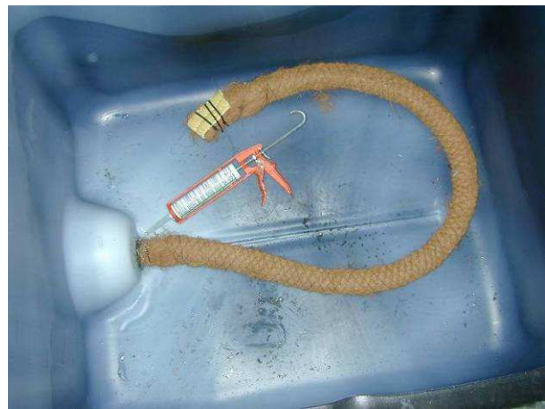
Fig 27: drain pipe at bottom of biofilter unit.
