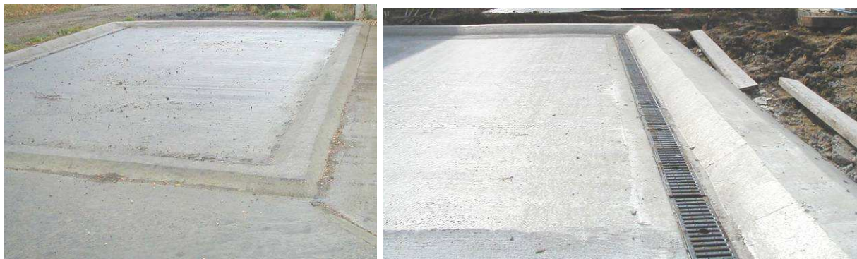
Fig. 16 & 17: Separate concrete filling and cleaning area which drains contaminated liquids to the bio purification system through a concrete path (left) or a drain grid (right) (source: ADAS).
